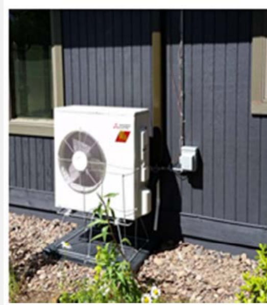
Ductless cold-climate air source heat pump
